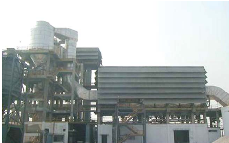
Figure 3. SO 2 Scrubber and Baghouse.
