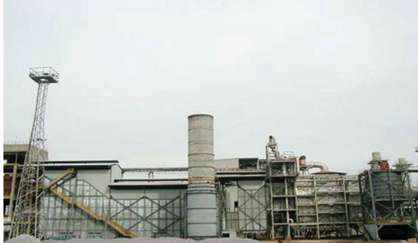
Figure 2. Pyroscrubber and Waste Heat Recovery Boiler.
